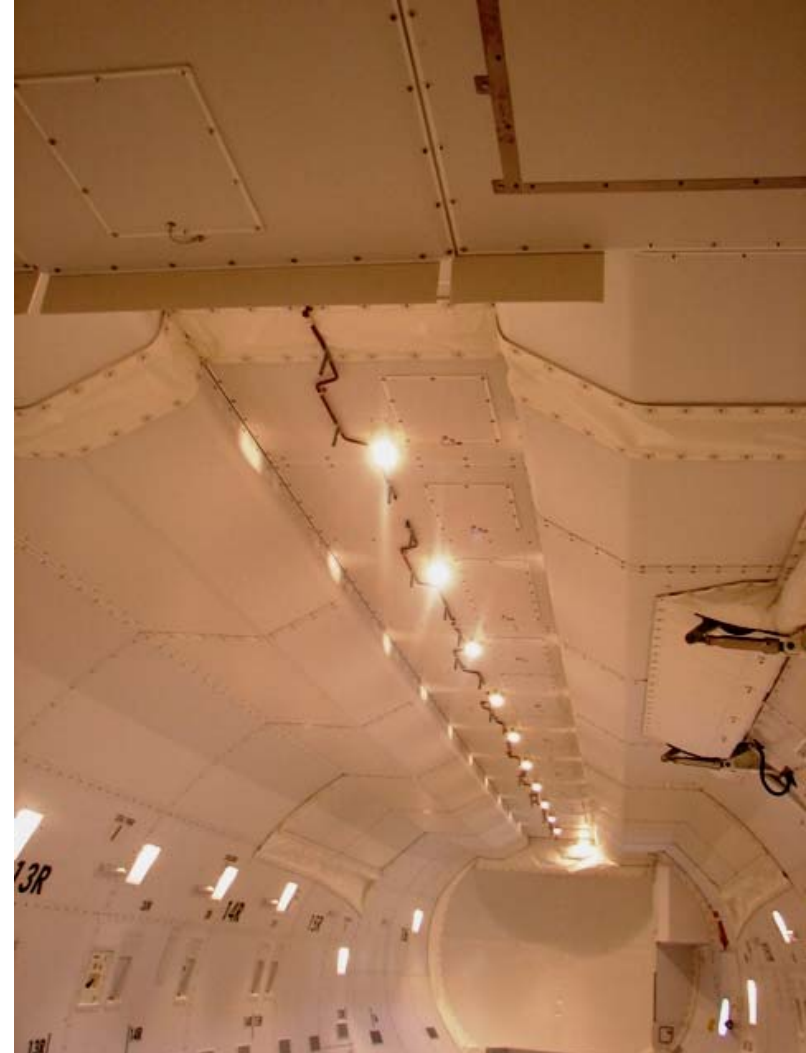
Smoke Detection and Halon System
